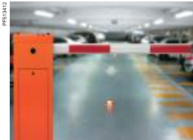
ATV12 controlling an access barrier
